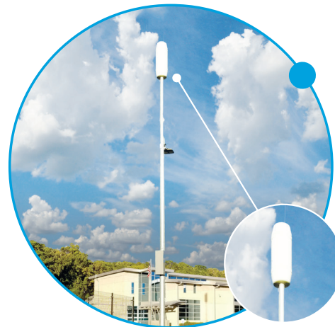
CAN DEPLOYMENT, KANSAS CITY, USA
